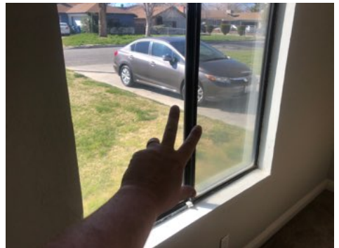
Missing lock- bedroom
