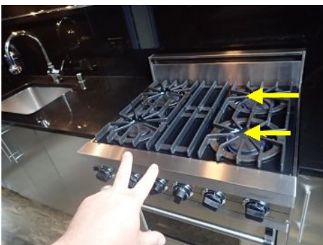
igniter not working properly
