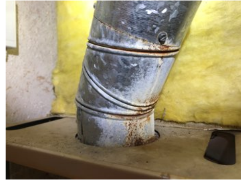
Rust/oxidation- have checked/evaluated
