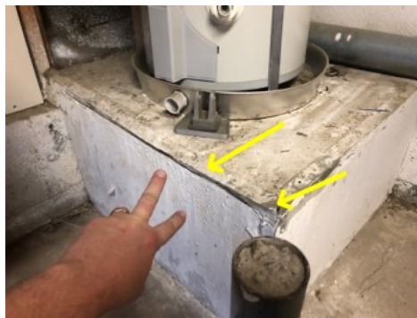
Damaged platform- have fixed
