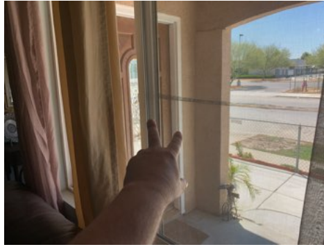
Won't lock/damaged screen
