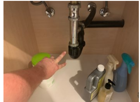
Leaking- master bath left sink
