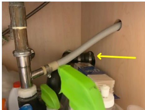
Washer drain- improper
