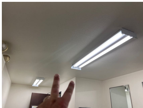
Missing covers - mens workshop bsth
