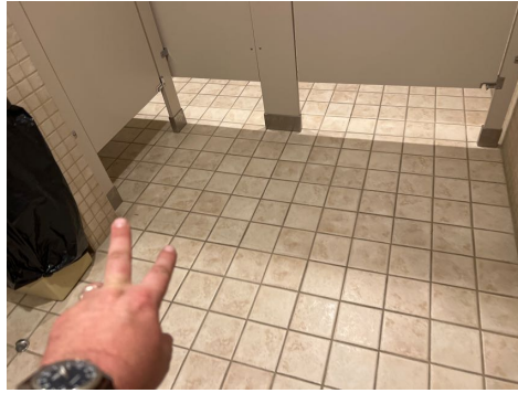
Women's upstairs restroom - cracked tiles
