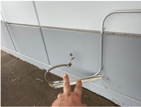
Left rear under pumps
