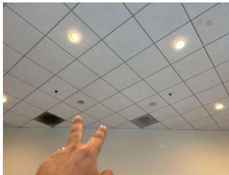
Not working - lobby
