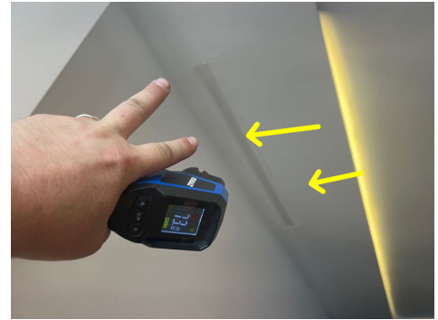
Vent covered, missing trim - primary bedroom
