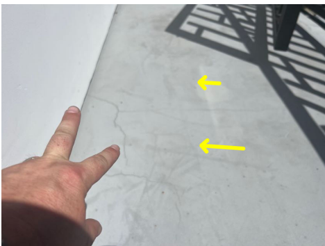
Cracked waterproofing - deck by pool
