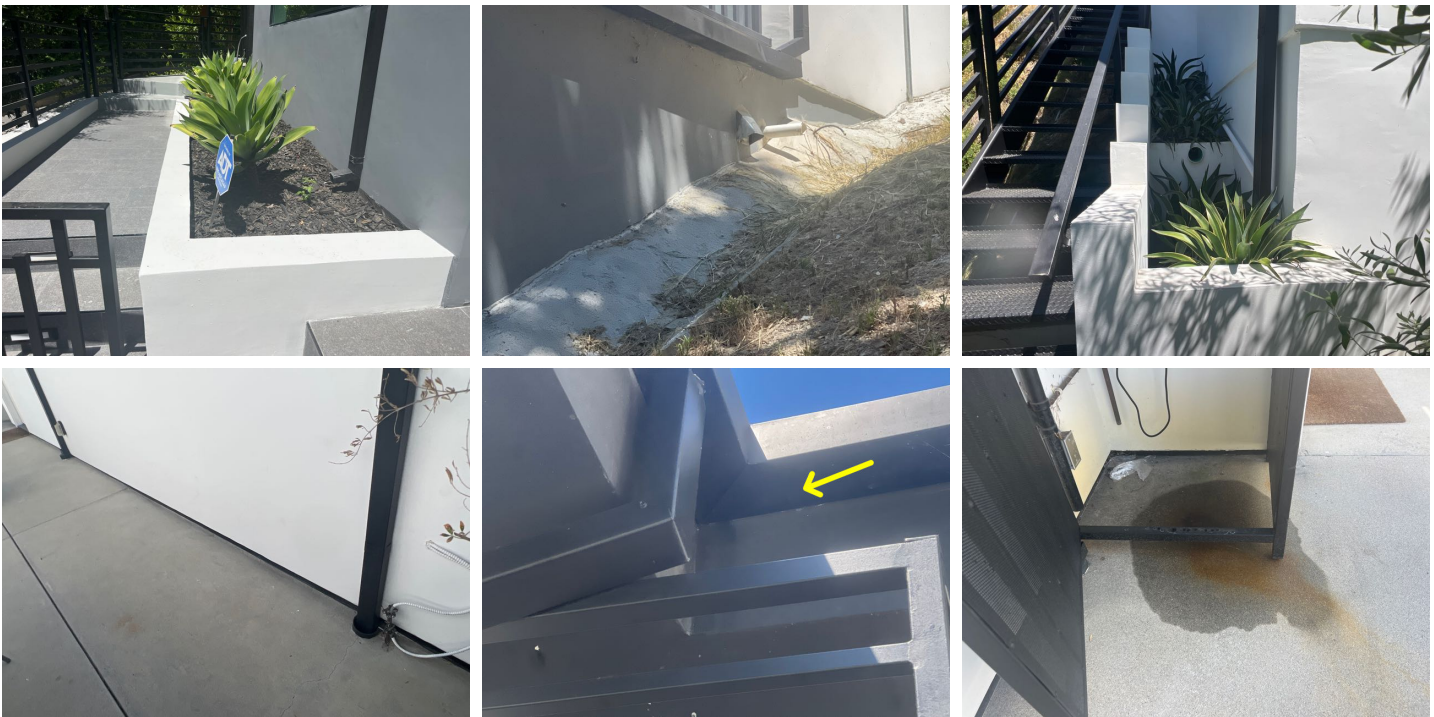
Gutter leaks- above water heater
