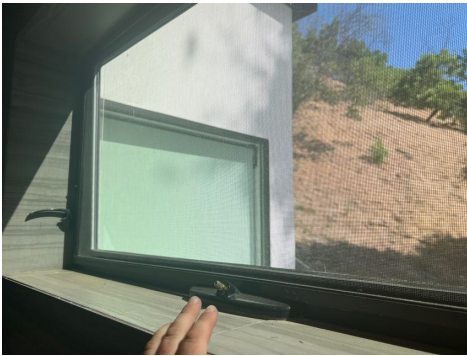
Missing crank- bath at bedroom
