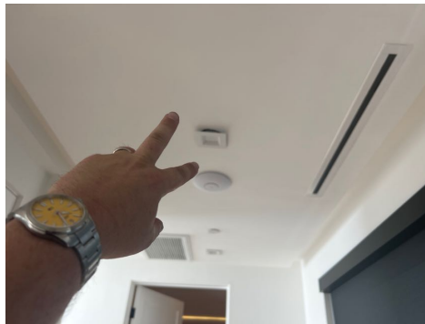
Loose light - upper level
