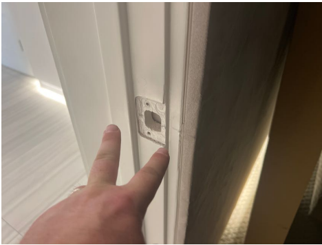
Missing strike plate - movie room
