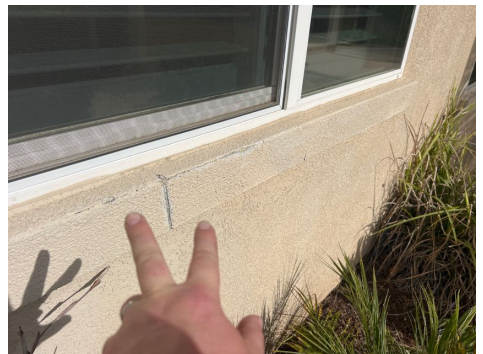
Damaged stucco molding - rear
