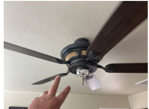
Missing light cover, light not working - primary
